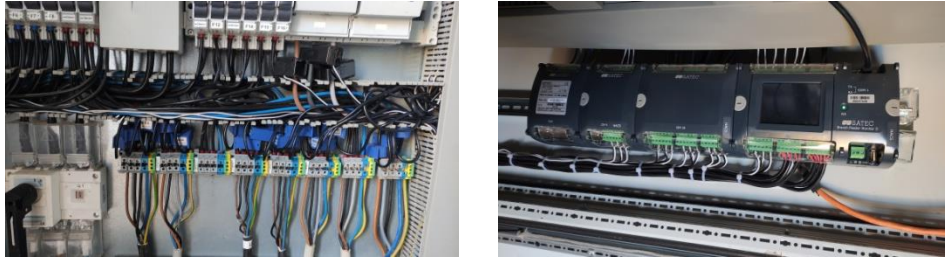
Figure 1. Installed energy consumption sensors in a pilot farm.
