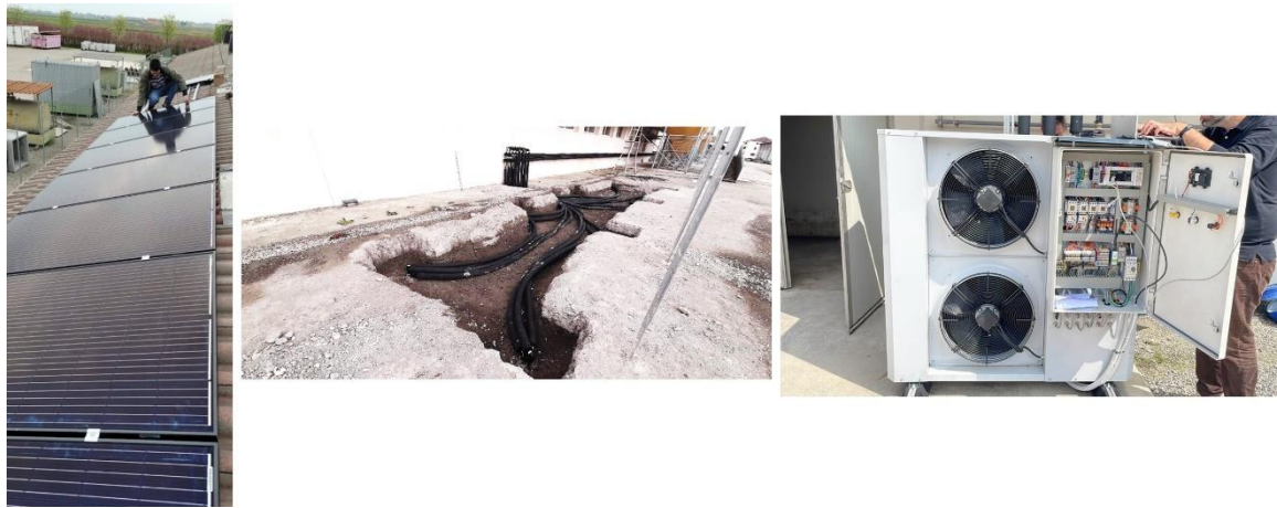
Figure 2. The PVT system (left), BTES system (middle), and HP (right) at GOLINELLI farm.
