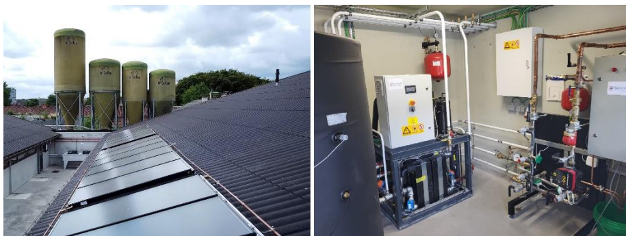
Figure 1. The PVT system (left) and HPs (right) at EV ILVO farm.
