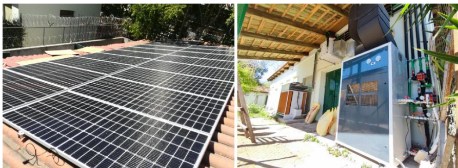
Figure 3. The PV system (left) and HP (right) at AUA farm.
