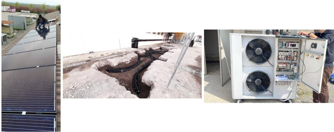
Figure 2. The PVT system (left), BTES system (middle), and HP (right) at GOLINELLI farm.
